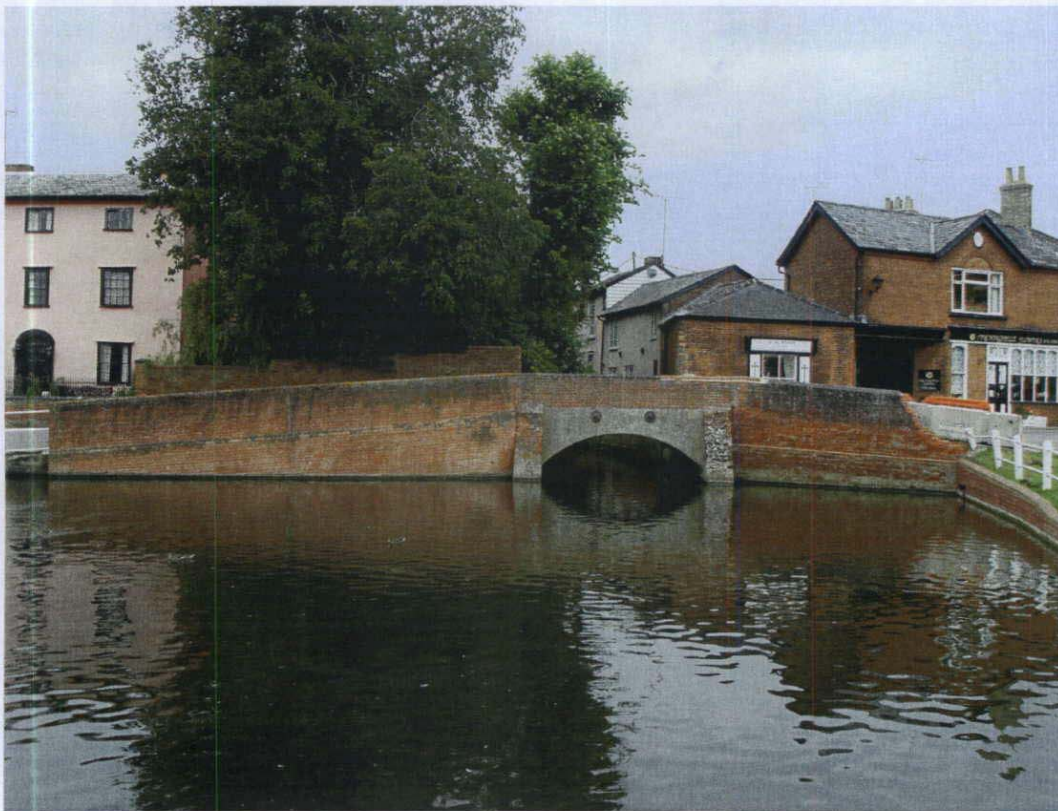
Photo No. 1 - General view of the brick arch bridge from South (upstream)
