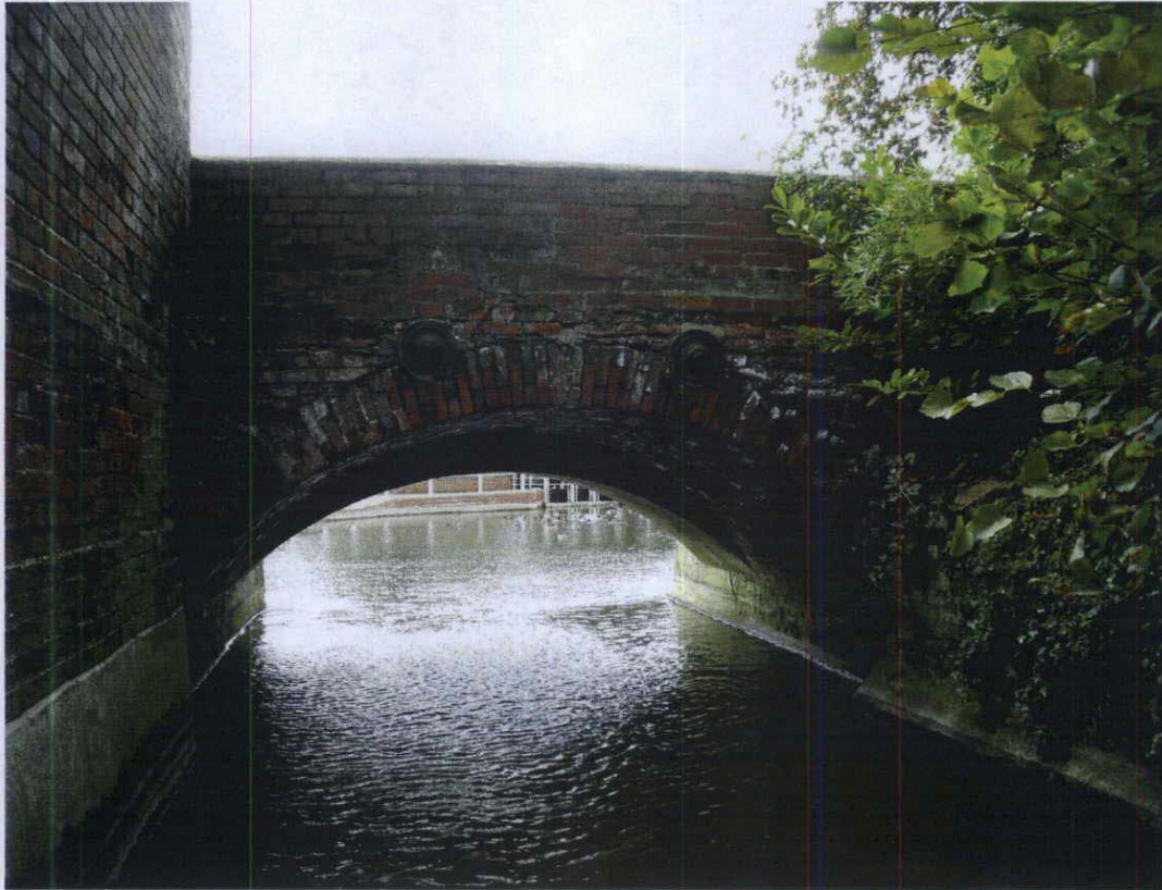
Photo No. 3 - General view of the brick arch bridge from North (downstream)
