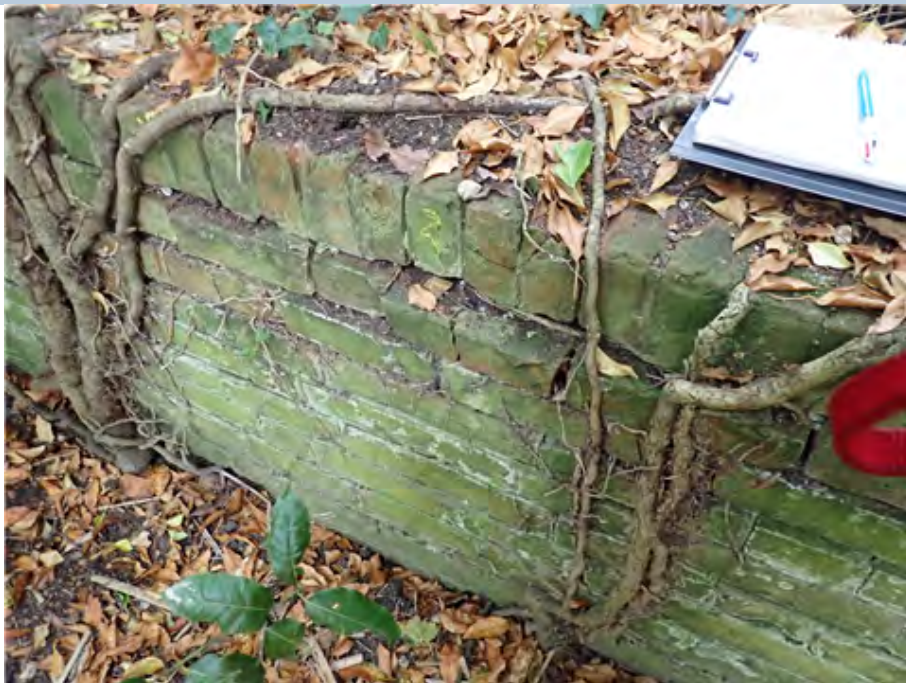
South West Wing Wall (west end) Brickwork displaced 30mm northwards.
