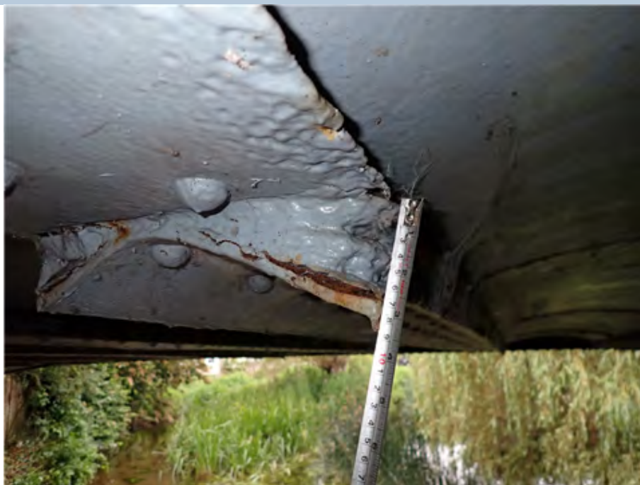
Transverse Beam Plate (East Side) Severe deflection due to corrosion up to 80mm. (6th beam in from the south)
