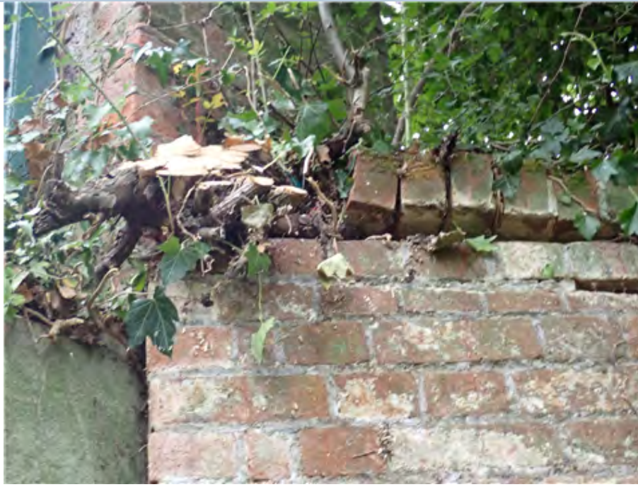
South West Wing Wall (east end) Tree root has pushed approximately 3no bricks off of top course.
