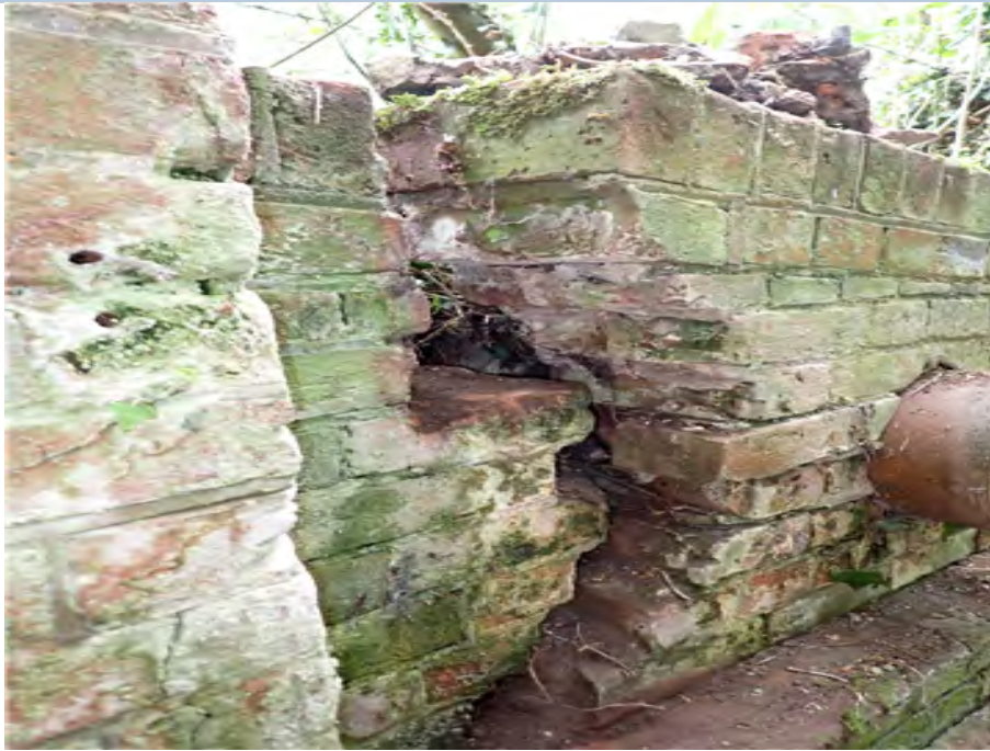
North East Wing Wall (looking north) Wing wall cracked through over full height, separated and significantly displaced.
