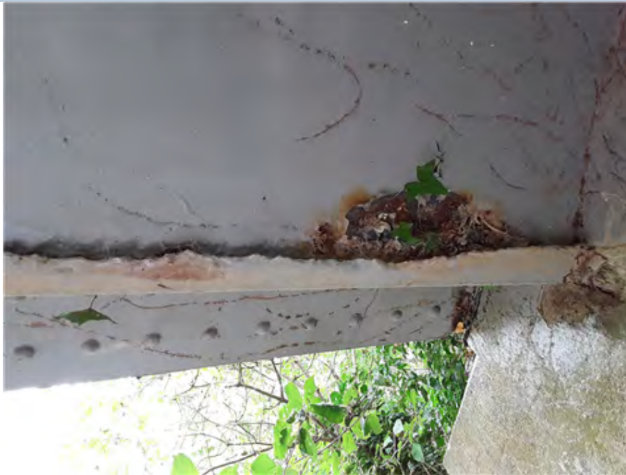
East Jack Arch at South End Section loss to jack arch hogging plate.
