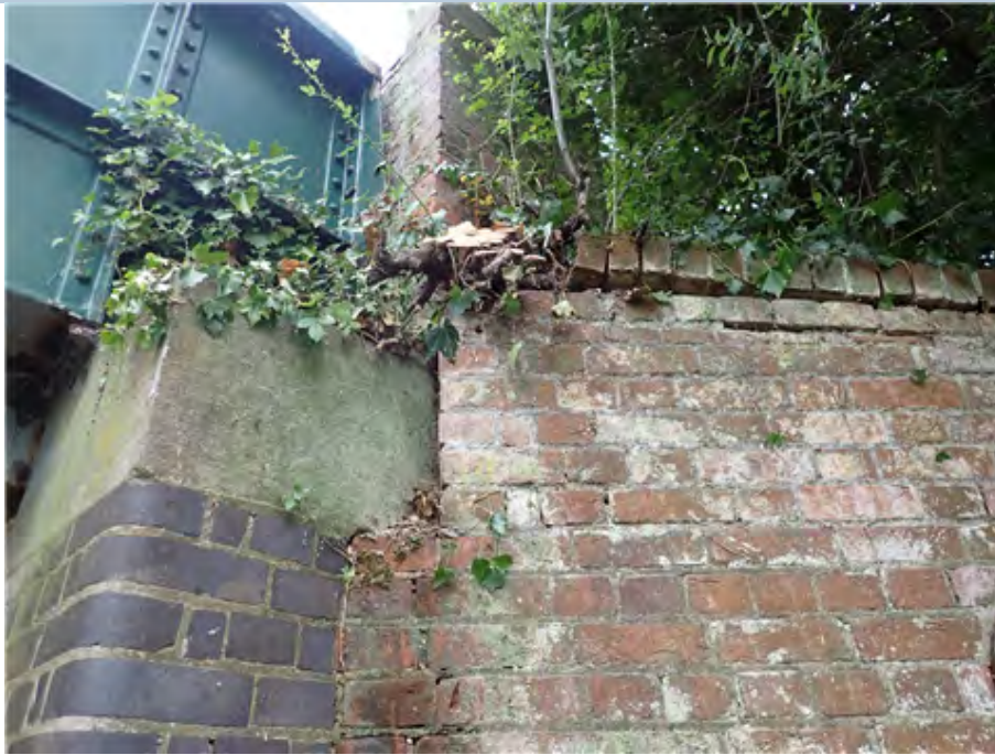
South West Wing Wall (east end) The top two brick courses were separated up to 60mm due to tree roots.
