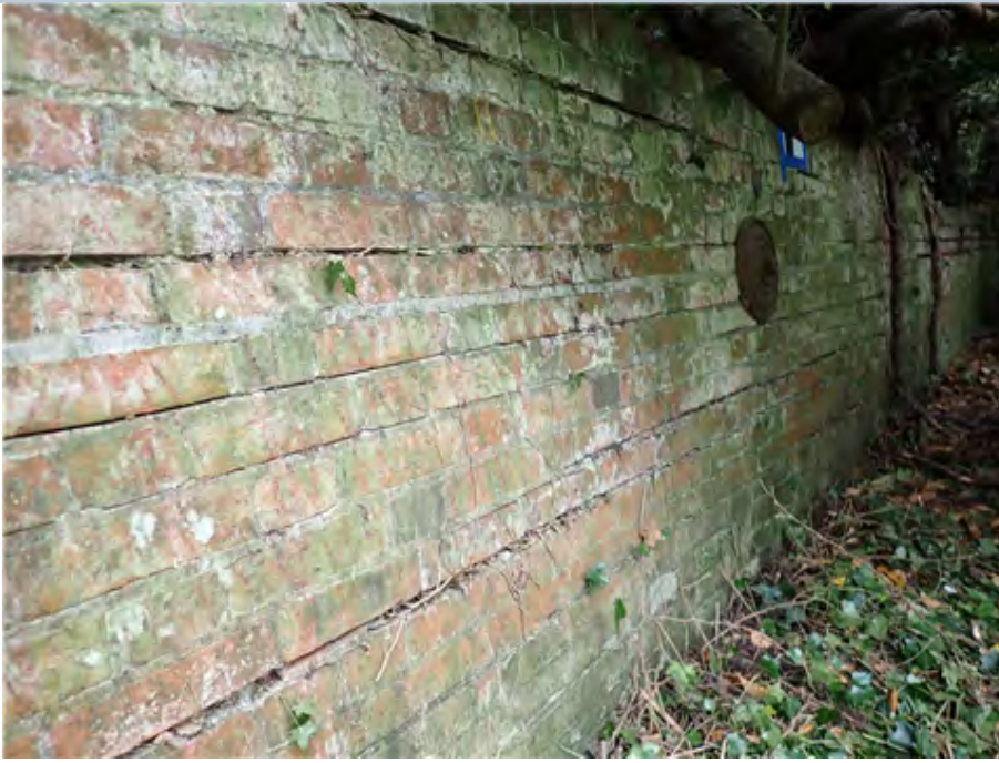
South West Wing Wall (looking west) Moderate bulging to midpoint of brickwork.
