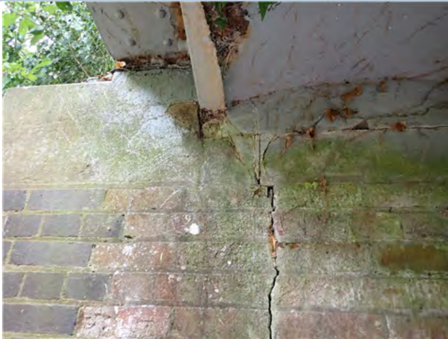
South abutment (east end) Spalling to jack arch concrete infill adjacent channel section (6m in from the west).
