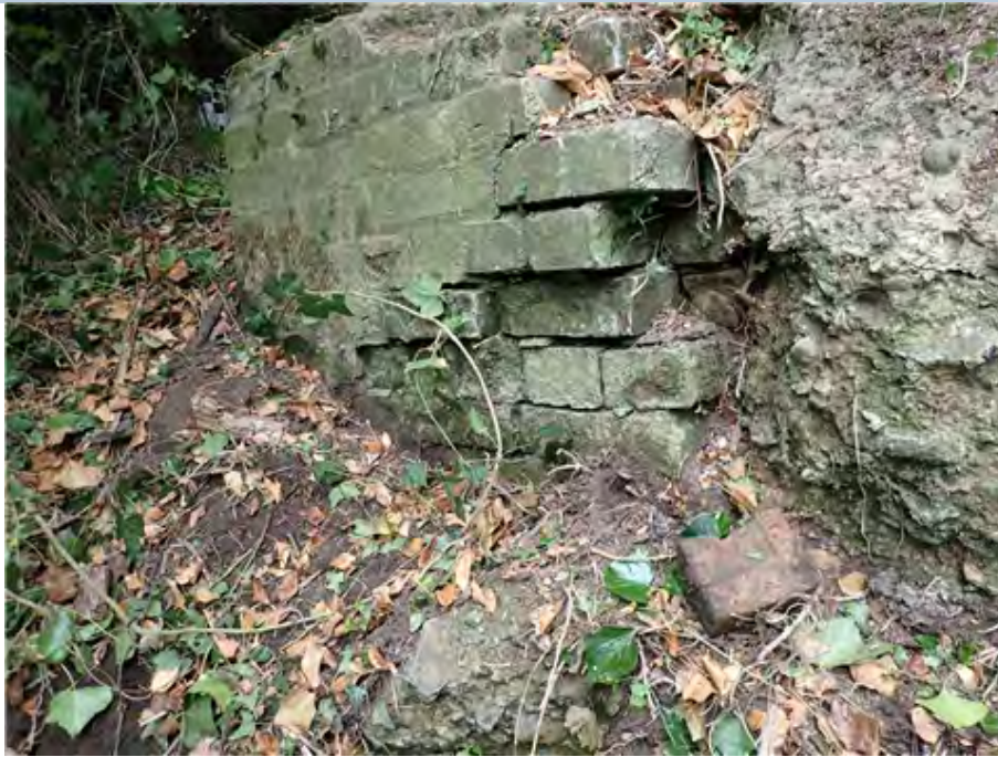
North West Wing Wall (lower section) Bricks breaking up and loose at south end of the wall.
