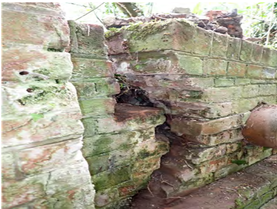
North East Wing Wall (looking north) Wing wall movement indicating possible movement of foundations.
