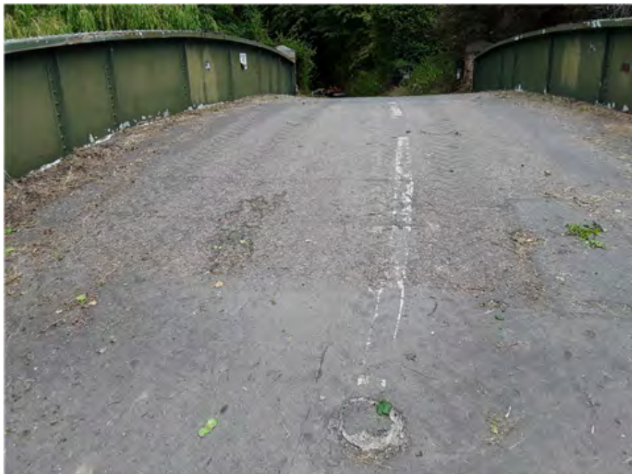
Carriageway Surface (looking north) Tracking to both carriageway lanes for 10m.
