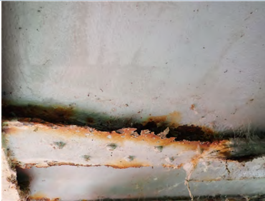
East Transverse Beam (At south end) Beam edges have corroded, causing section loss both in width and in thickness. (3rd beam in from the south)
