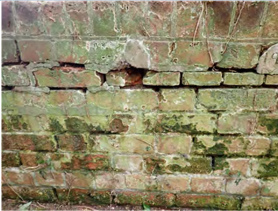
North East Wing Wall Area of bricks breaking up to upper section.
