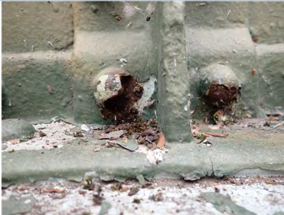
East Edge Girder Stiffener Rivets (East Face) (south end) Corroded rivet heads.
