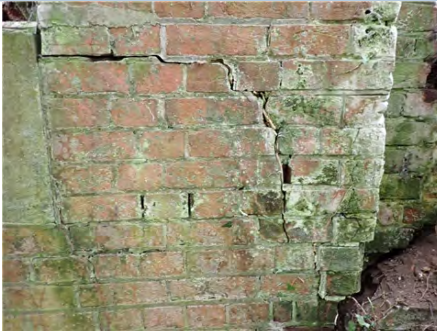
North East Pilaster (east face) Stepped diagonal crack extending from bearing stone to wing wall open 3.5mm with vegetation roots growing in the gap.
