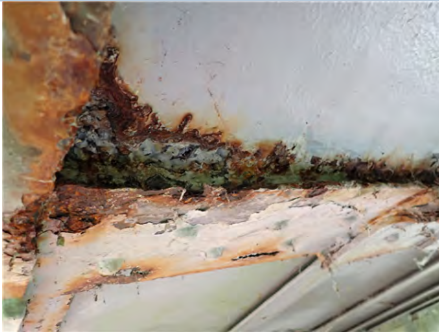
East Jack Arch Hogging Plate Edge (at south end)
