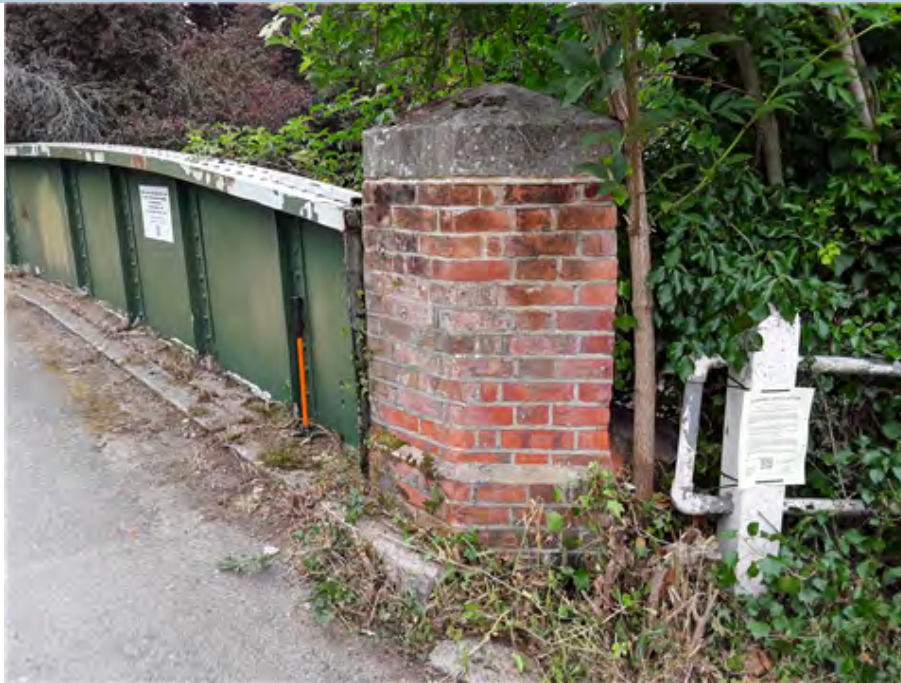
South East Pilaster (south face) Tree growing adjacent SE corner of pilaster.
