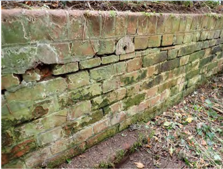
North East Wing Wall Pointing loss to upper section between bricks to a maximum depth of 20mm.
