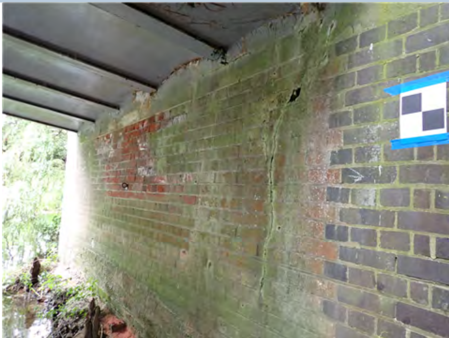
North Abutment (looking west) Full height crack indicating possible movement of foundations.
