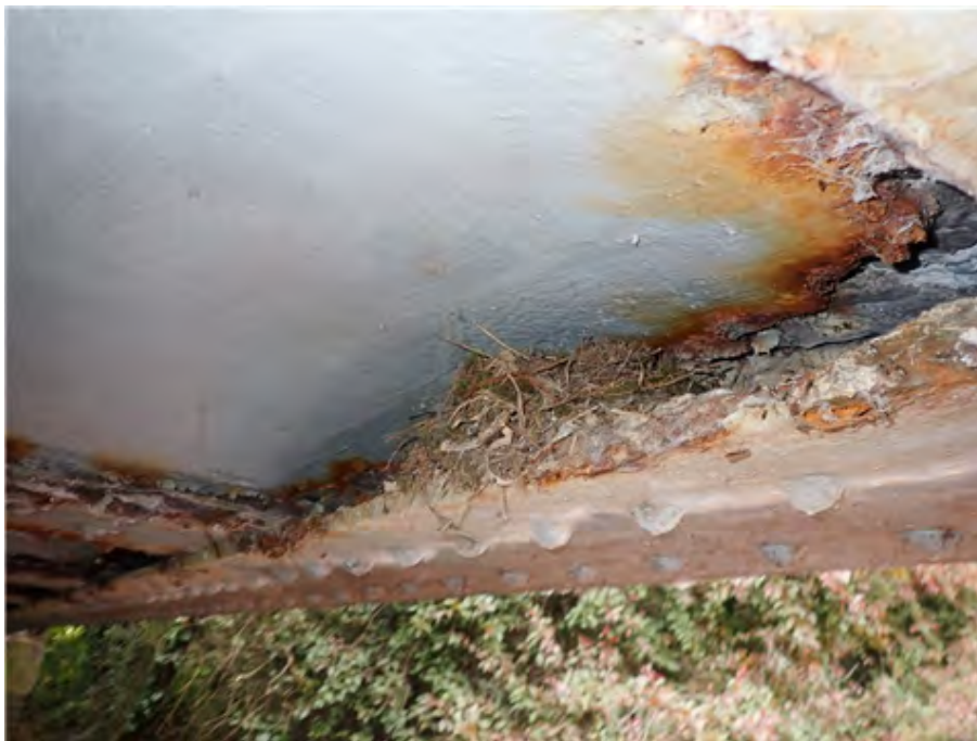
East Edge Girder Bottom Flange Disused birds nest on east edge girder inner bottom flange between the 2nd and 3rd transverse beam from the south.
