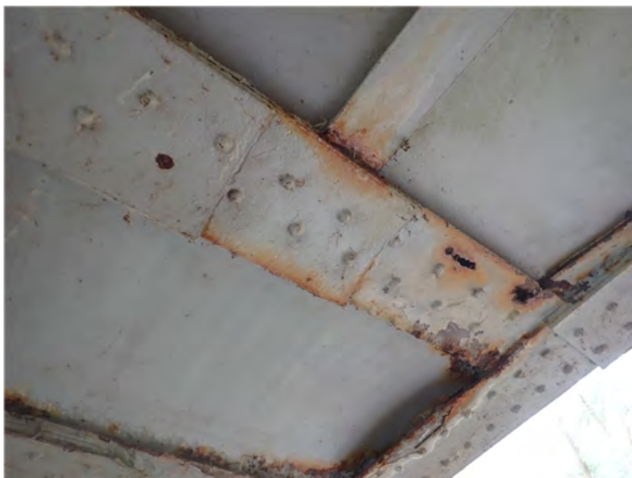
Riveted Transverse Beam Plate (East Side) Missing rivet due to deflection. (1st beam in from the south)
