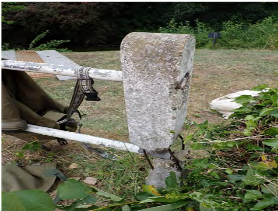
South East Approach Rail Concrete post broken at lower rail joint being held together by reinforcement. D end cap missing.
