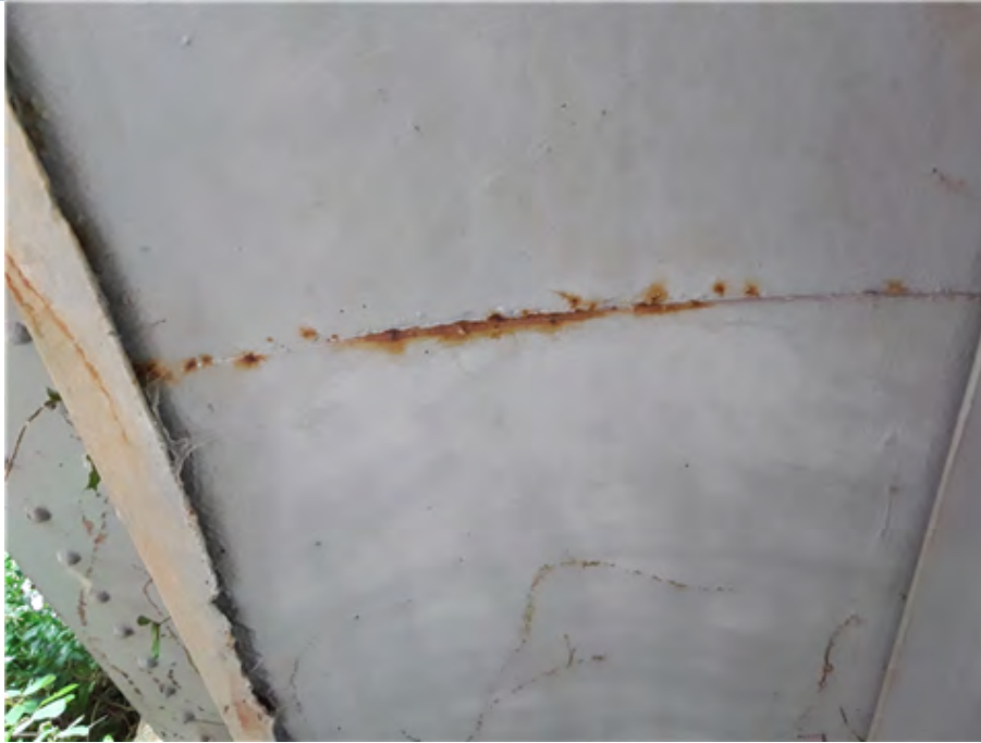
East Jack Arch Hogging Plate Joint (at south end) Minor corrosion of hogging plates at joint.
