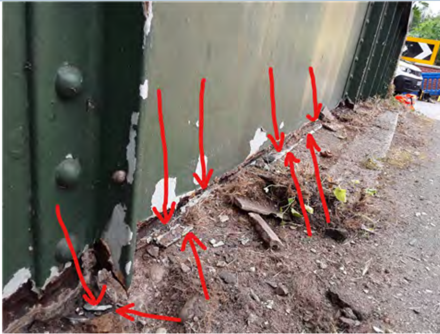
East Internal Topside Edge Girder (midpoint) Sealant broken up and cracked.
