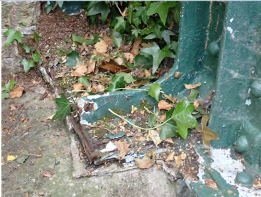
South East Bearing Plate Corrosion to bearing plate.
