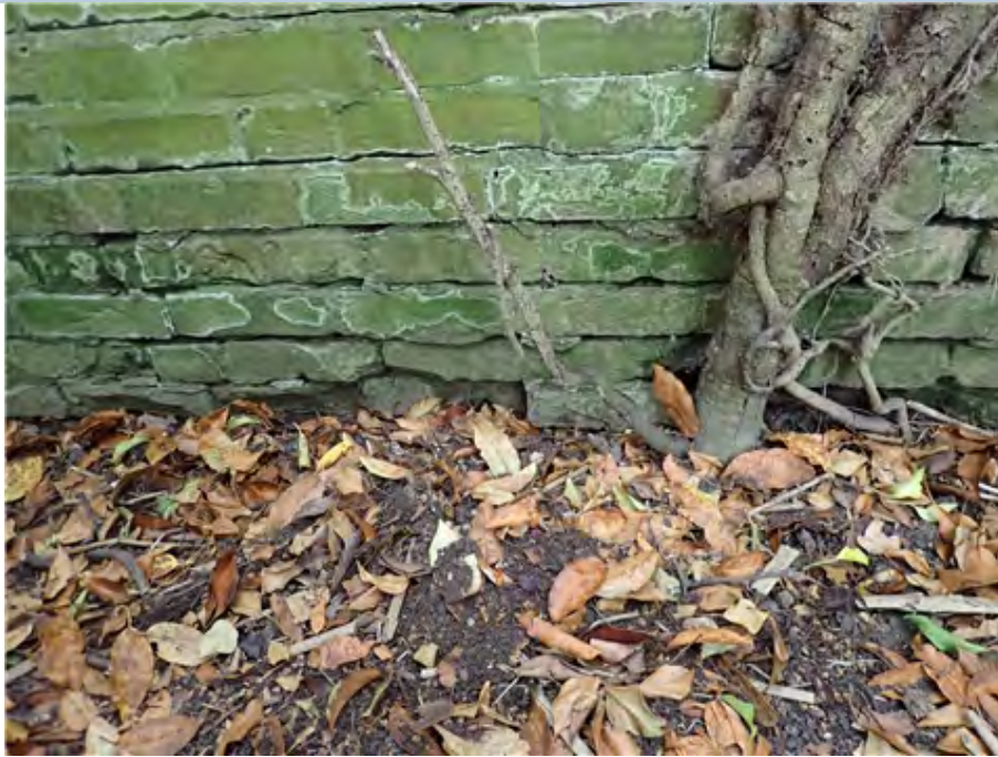
South West Wing Wall (west end) Brickwork breaking up at bottom of wing wall to a maximum depth of 40mm.
