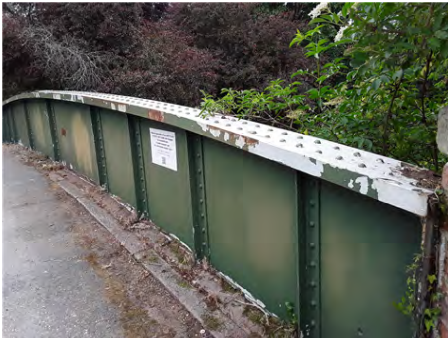
East Edge Girder Top Flange (looking north) Protective paint top coat flaking.
