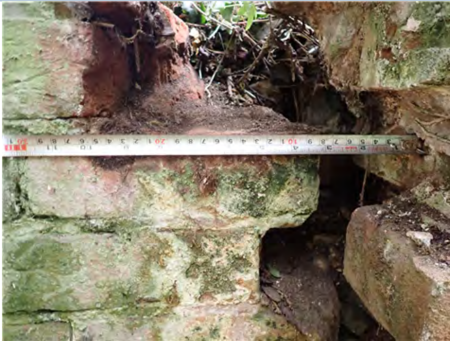
North East Wing Wall (looking west) Gap separation maximum 250mm at widest part.
