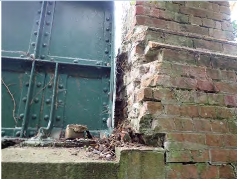
North East Pilaster (south east corner) Bricks broken up, loose and missing.
