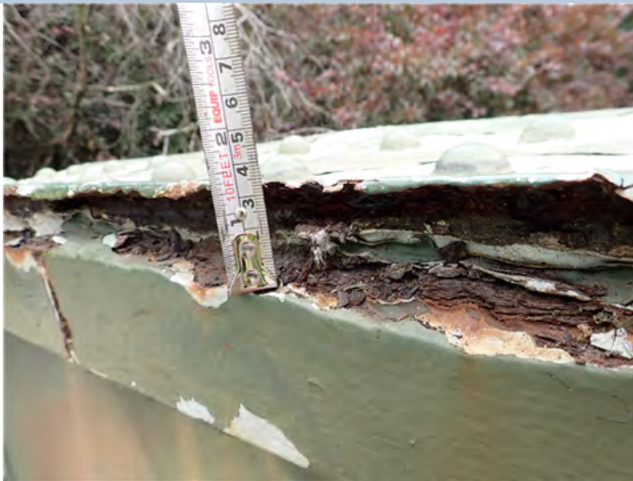
East Edge Girder Riveted Splice Plate Severe corrosion leading to deflection of up to 35mm.
