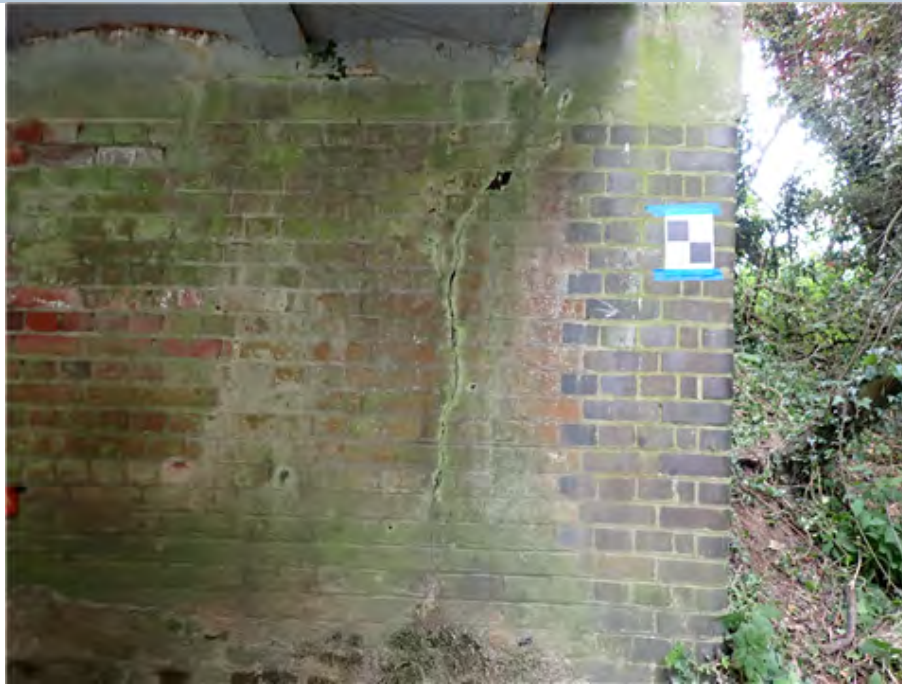
North Abutment (east end) Vertical crack to north abutment.
