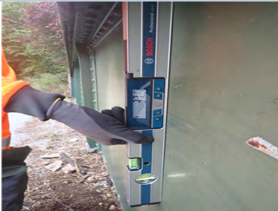
East Edge Girder Web (midspan) Rotation of 37mm/m. Overall Girder rotation of up to 65mm full height.
