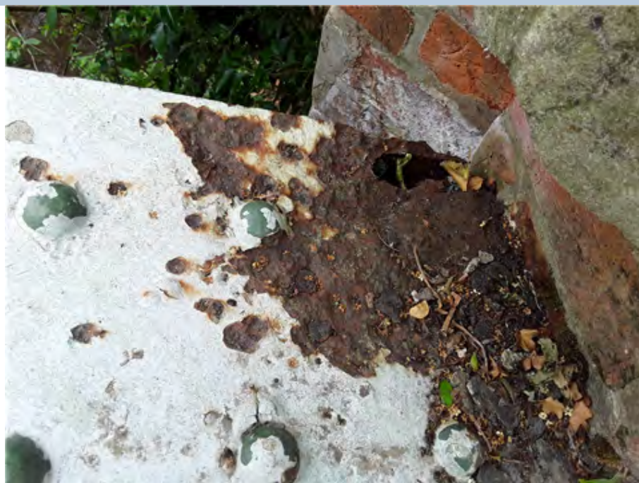
East Girder Top Flange (south end) Severe corrosion leading to section loss.
