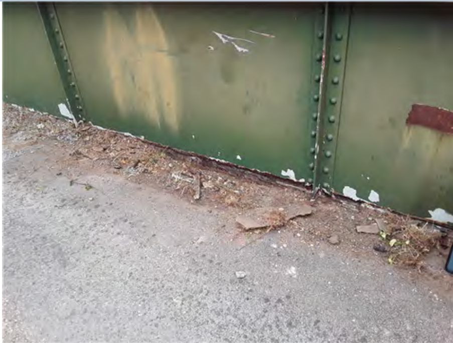
East Carriageway (midspan) Concrete edge fillet broken up.
