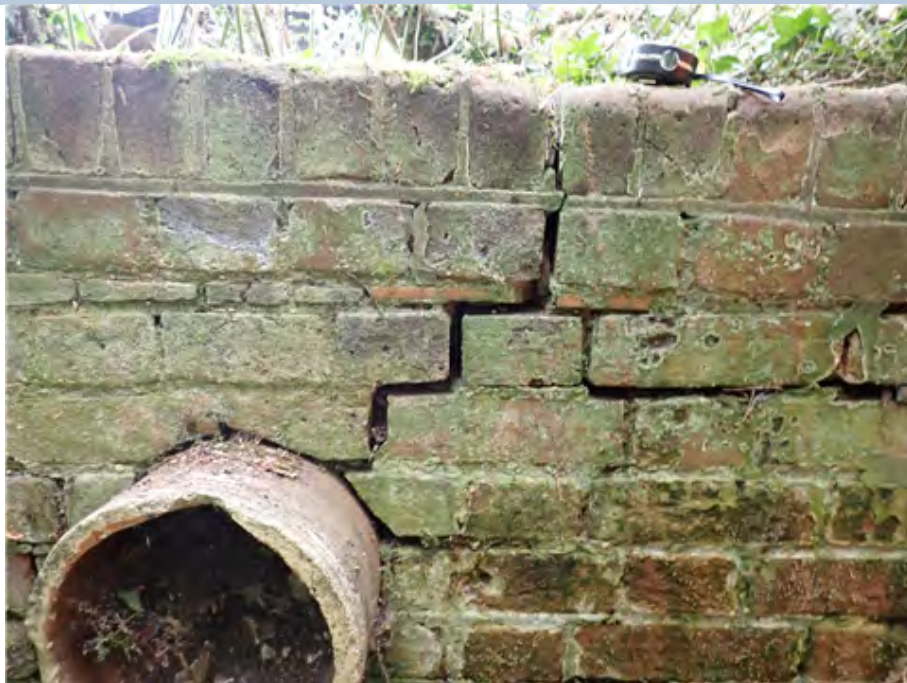
North East Wing Wall Stepped crack open 15mm, extending from near top of the wall to the top of the redundant drainage outlet.
