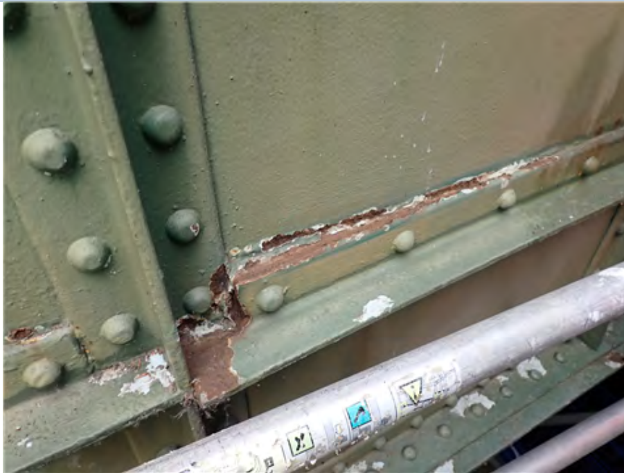
East External Edge Girder (south side) Corrosion to the edge girder web and rivet plates of the T stiffeners.
