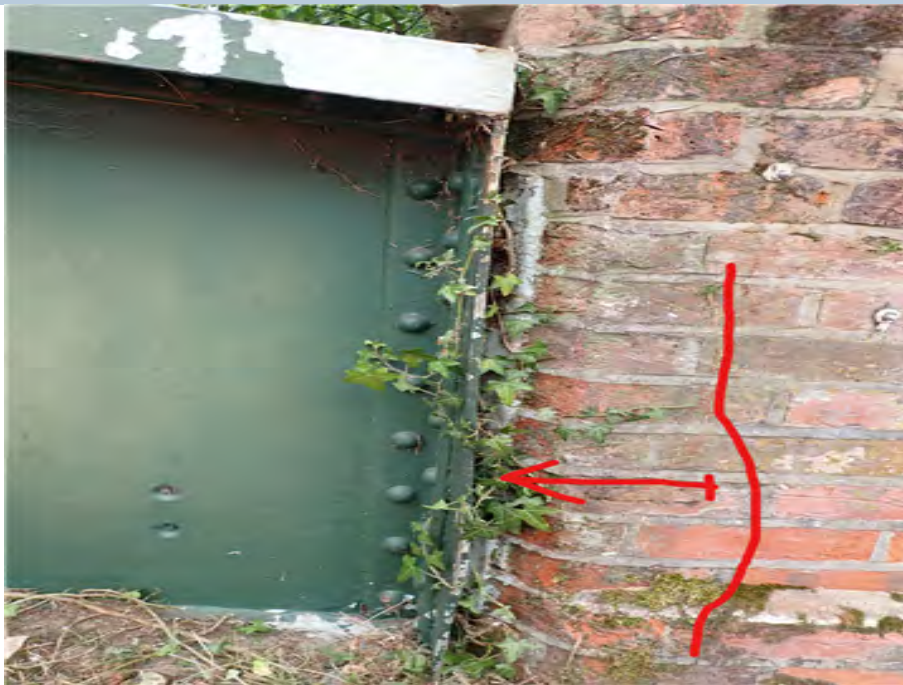
East Internal Edge Girder (south end) Deformation of end plate of 15mm due to impact damage.
