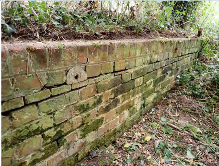
North East Wing Wall Moss growing on brick surface.
