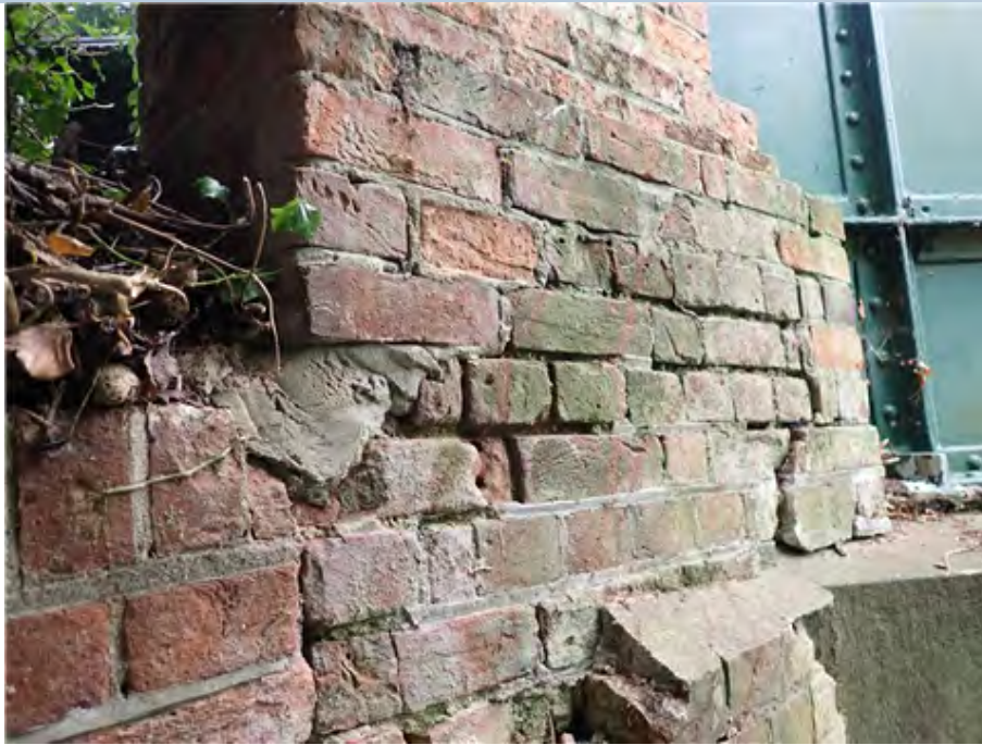
North West Pilaster (west face) Pointing loss of up to 10mm in depth between bricks.
