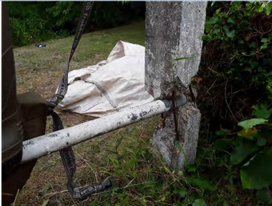
South East Approach Rail Concrete post broken at lower rail joint being held together by reinforcement.
