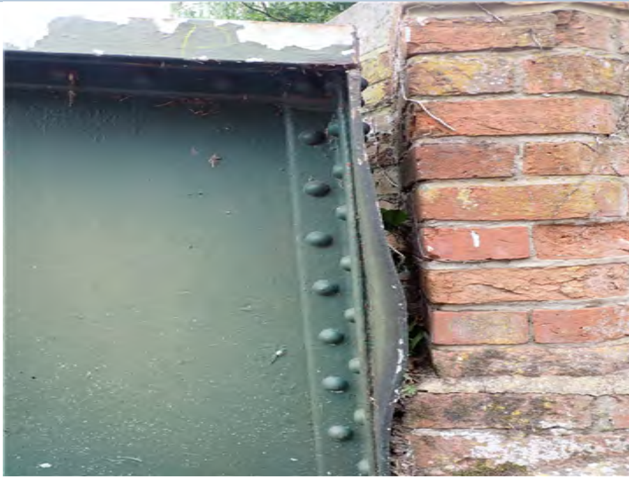
West Internal Edge Girder (north end) Deformation of end plate of 30mm due to impact damage.
