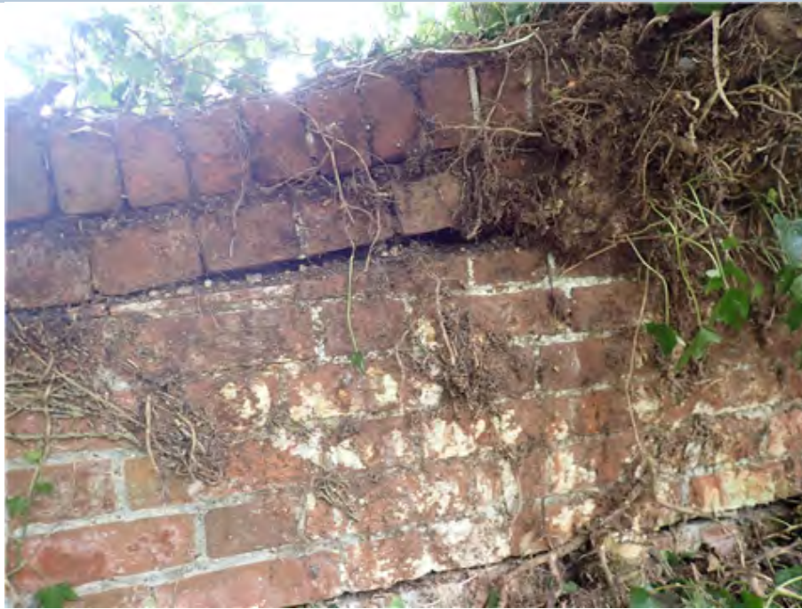
South East Wing Wall Tree root damage to wing wall 4m in from the west,
