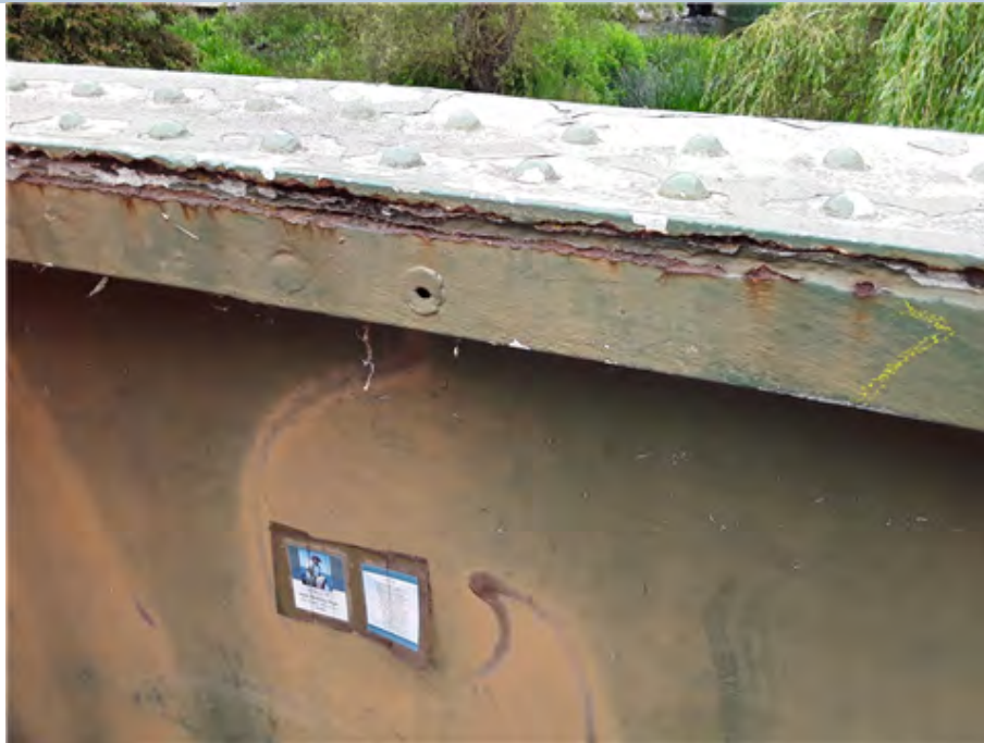
Western Girder (East Face) Missing rivet.
