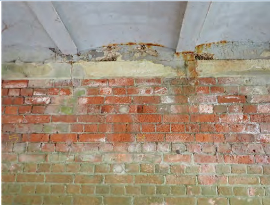
South Abutment Weathering to brick faces
