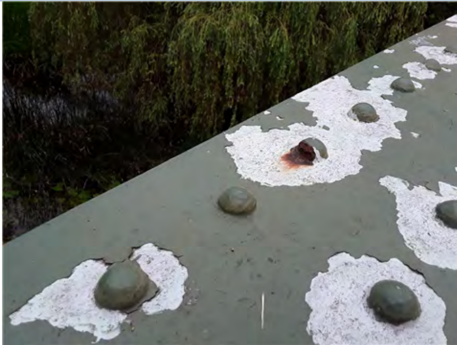
West Edge Girder Top Flange (south end) Rivet corroding away with protective paint loss to girder.
