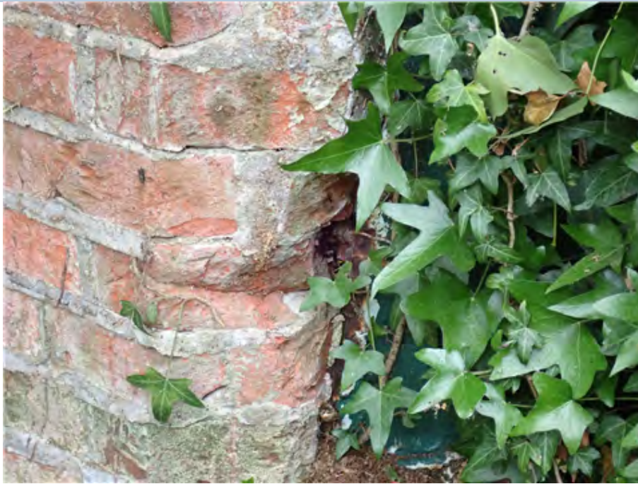
South East Pilaster (NE corner) Bees nest in pilaster void just above abutment.
