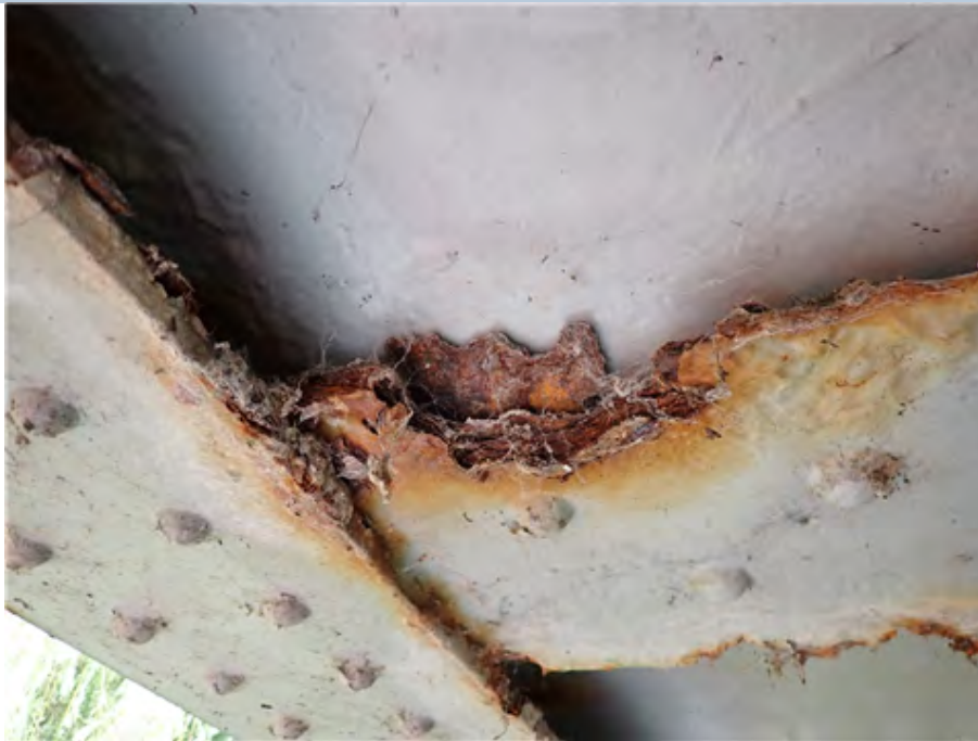
West Transverse Beam (at north end) Severe section loss and corrosion. (6th beam in from the south)
