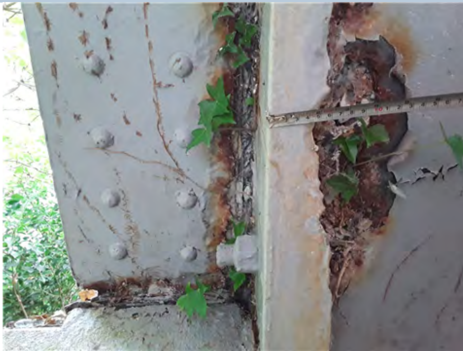
East Channel Section at South End. Section loss of up to 35mm to bottom flange of channel section.
