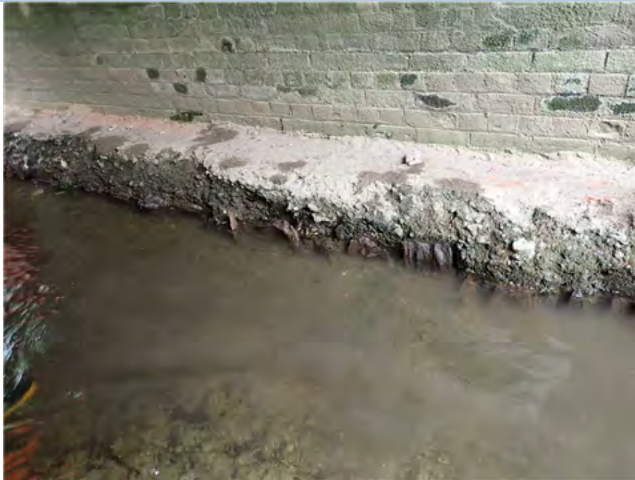
River Bed in front of South Abutment. Broken timber posts at river bed edge.
