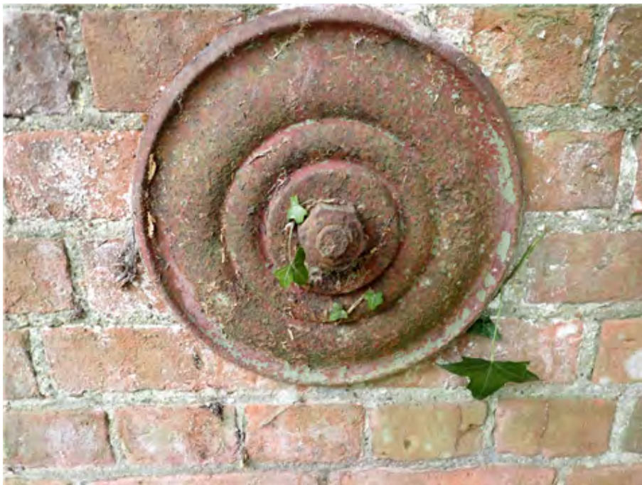
South West Wing Wall (east end) Pattress plates and tie rods are heavily corroded.
