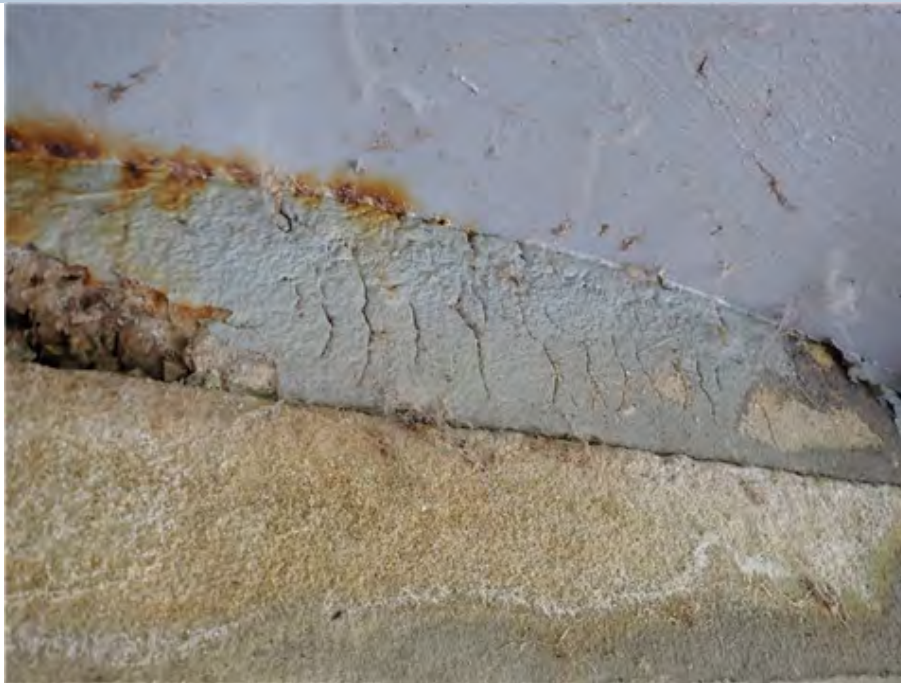
South Abutment (west end) Jack arch infill has shrinkage cracks.
