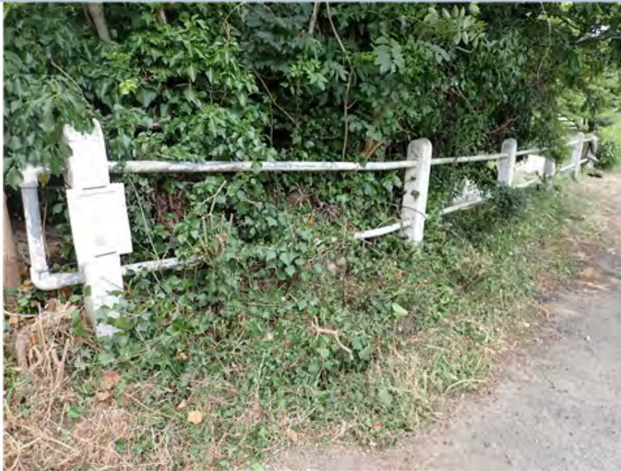
South East Approach Rail Protective paint top coat chipped and flaked on railings and concrete posts.
