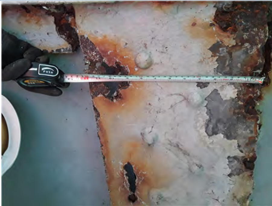
East Transverse Beam (At south end) Severe section loss and perforation due to corrosion. (1st beam in from the south)
