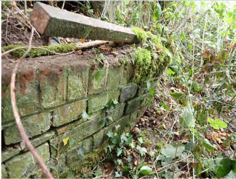
North East Wing Wall (looking north) Wing wall leaning due to adjacent tree.
