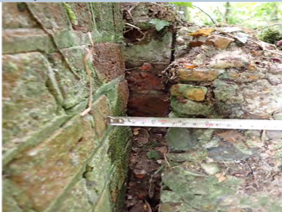
North East Wing Wall (looking north) Concrete plinth at the base of wing wall displaced by 60mm.
