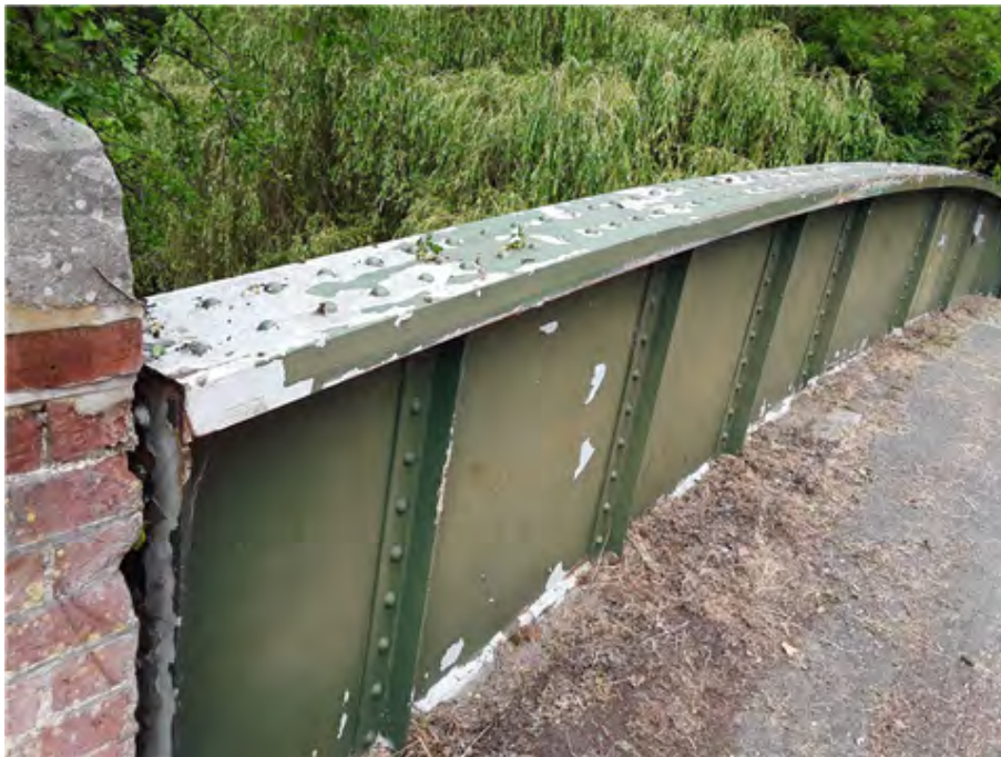
West Carriageway Edge Grasses and weeds growing along between edge kerbing and edge girder.
