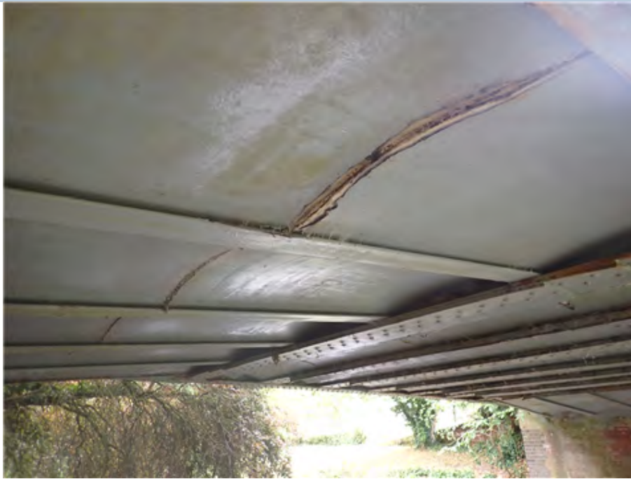
Jack Arch at West side at north end Jack arch misaligned 30mm to the west jack arch at north end.
