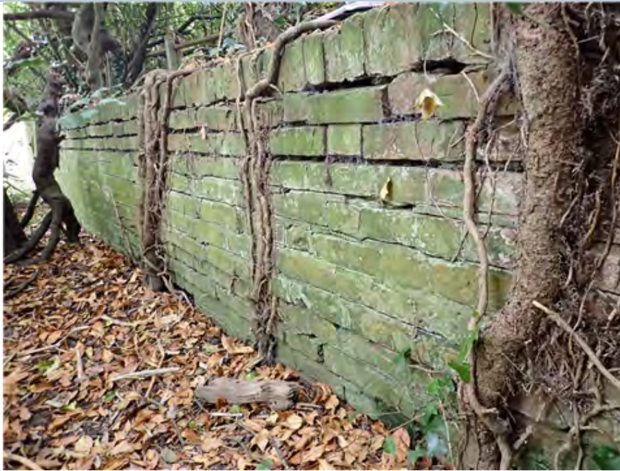
South West Embankment (west end, looking east) Tree roots growing on wing wall and embankment.
