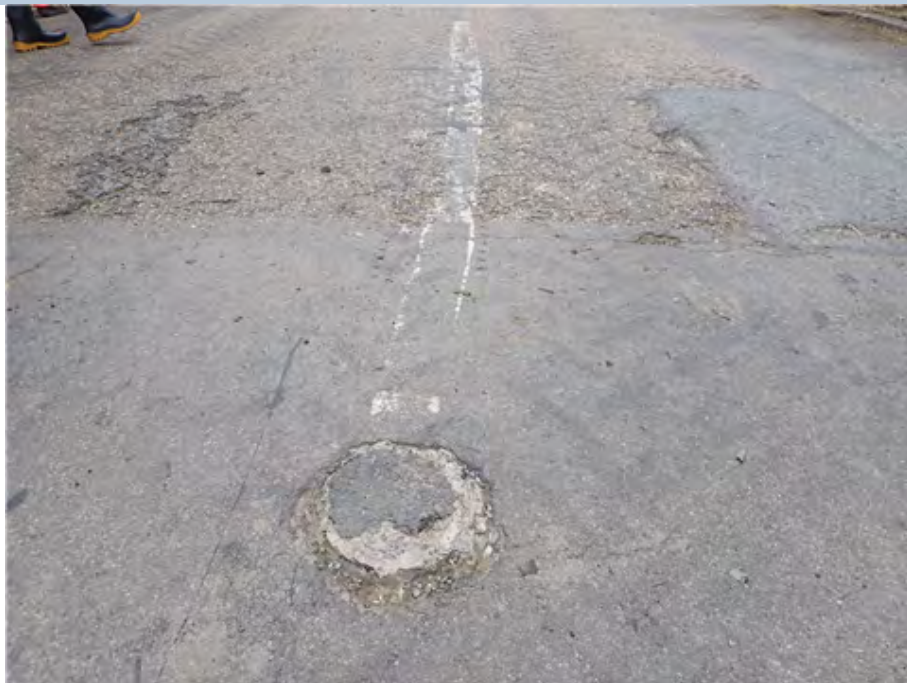
Carriageway Surface (south end) Shallow potholes 3no. to south end.
