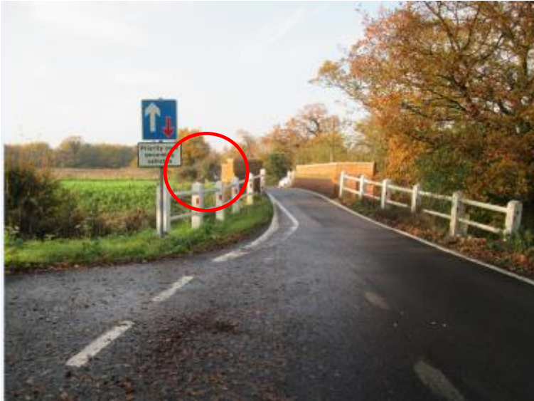
Image 2 – See through between parapet and sign
