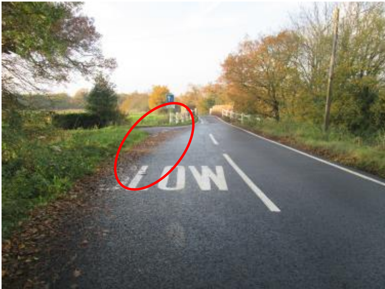
Image 1 – Northbound approach to bridge (road narrows on nearside; also see detriutus on nearside)
